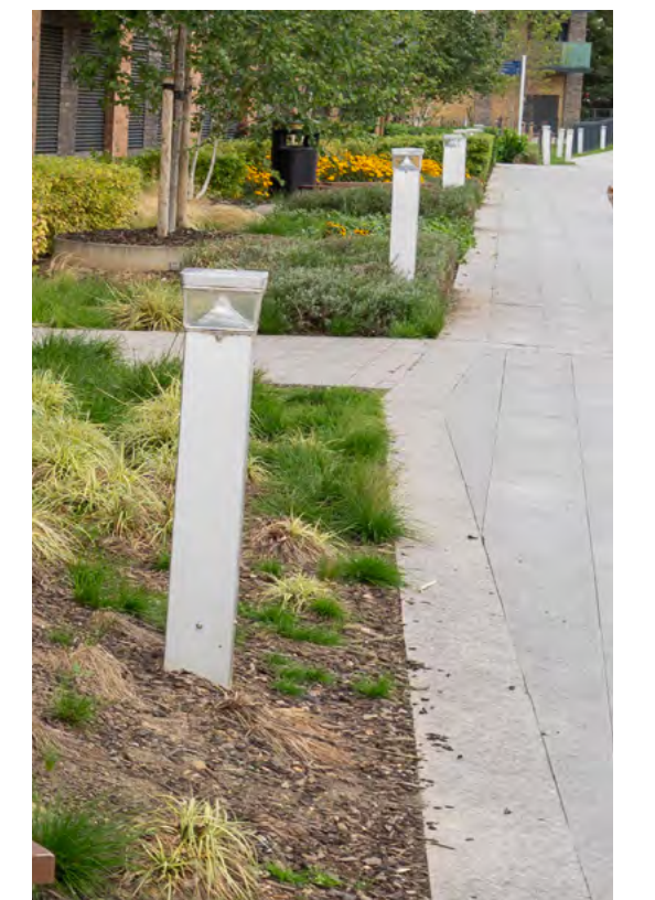
Figure 99. Stainless steel light bollards
