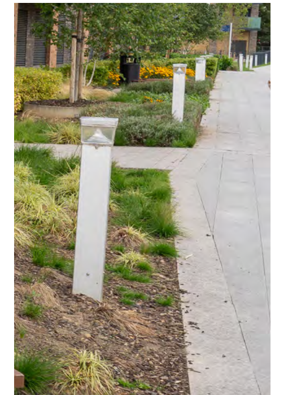
Figure 99. Stainless steel light bollards
